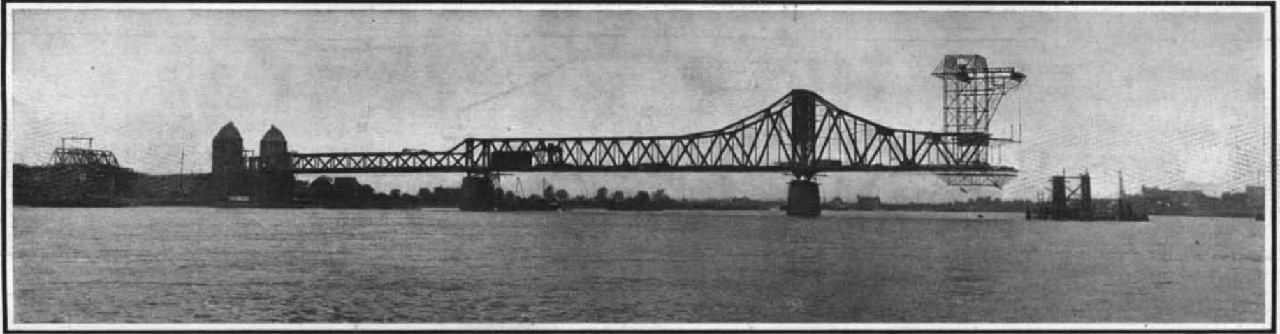
Highway Bridge Across the Rhine Between Ruhrort and Homberg, Showing Method of Erection by Overhang.
