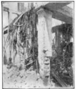
Effect of fire on reinforced concrete structure. A so-called "fire-proof" building. Name and location of above building sent on request.
