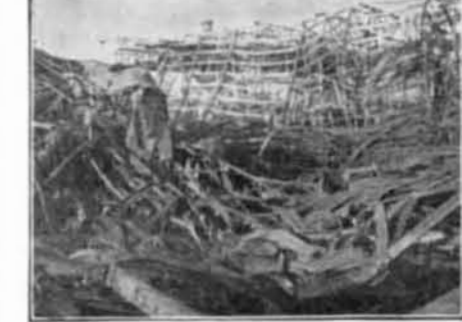
Effect of fire on unprotected steel—so-called "fire-proof" construction. Name and location of above building sent on request.
