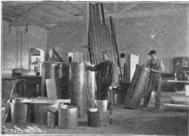
In the Pipe Room.
