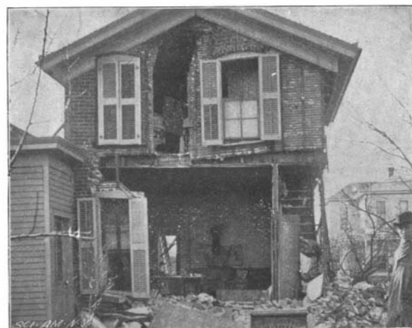
REAR OF HOUSE WRECKED BY GAS EXPLOSION.
