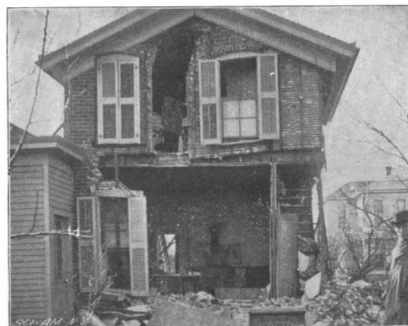
REAR OF HOUSE WRECKED BY GAS EXPLOSION.
